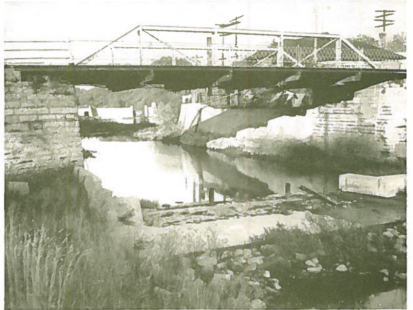
Highway Bridge at Mitchell—a new bridge with a 75-foot clear span would be erected here.
