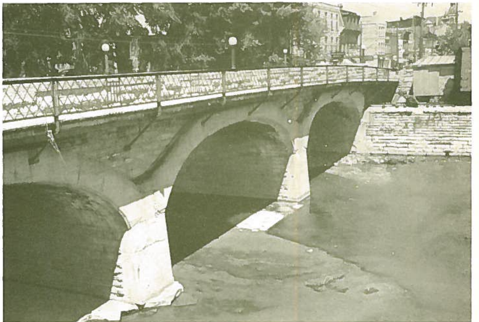
Queen St. Bridge—limited opening at this bridge further aggravates the flood conditions.
