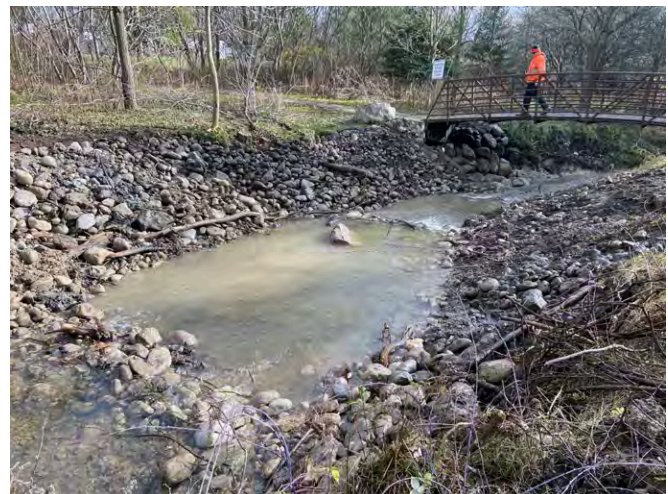
Downstream of the bridge (after): The bank has been shaped to a gentler slope and stone with filter cloth underlay was added.
