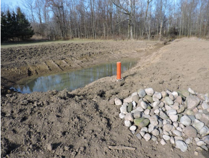
This marsh collects water flowing overland from a wooded area. A shallow scrape creates open water. A standpipe inlet and overland swale provide a safe outlet for large runoff events. Trees and shrubs were planted this spring to further enhance the new wetland.
