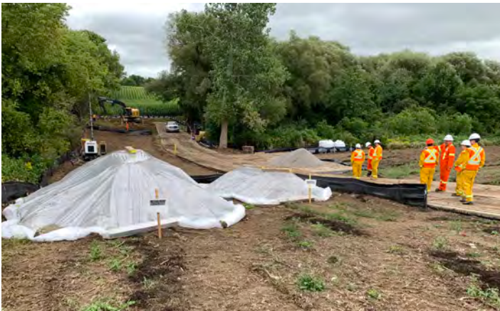
The Sun Canadian Pipeline site had temporary topsoil stockpiling under tarps, and construction matts to protect the farm field from heavy equipment.
