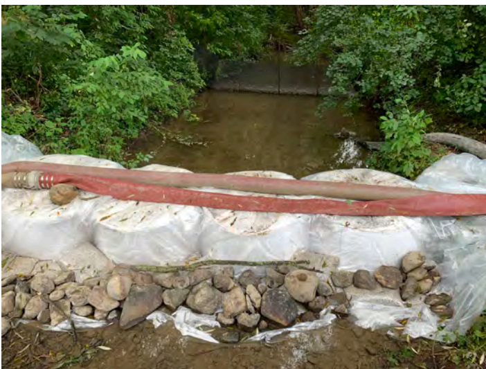
A fish protection screen is visible upstream of a coffer dam, which is being used to temporarily dewater a short section of the creek, in anticipation of pipeline remediation.
