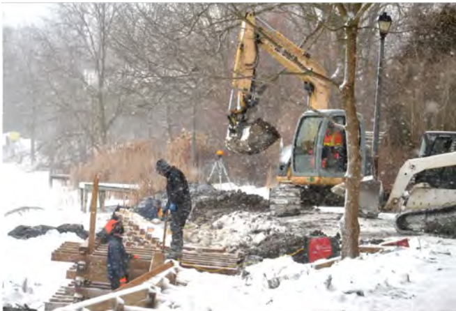
Staff and contractors with the Upper Thames River Conservation Authority worked to complete construction on a number of shoreline improvements along Lake Victoria's north shore in Stratford Friday morning. Improvements include making a 60-metre stretch of the city's north-shore pathway more accessible, constructing wooden cribbing and reinforcing the shoreline with rocks to prevent further erosion, and building a kayak and canoe launch closer to the water to make it easier to get in and out from shore. Galen Simmons/The Beacon Herald/Postmedia Network
