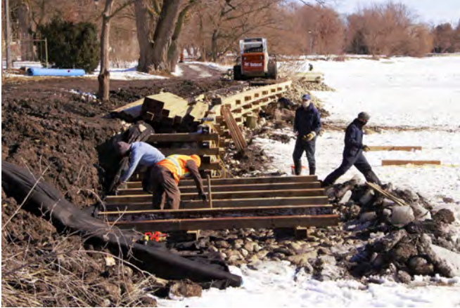
The accessible canoe/kayak launch and erosion control are constructed of a timber cribwall with underwater rock shoals.
