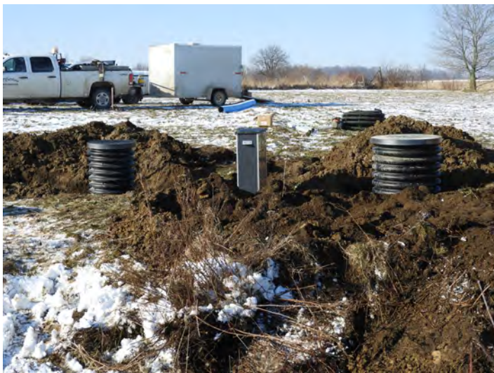
A control box (in the centre) diverts water from the underground field tile into two filter units of different sizes, to test their ability to remove phosphorus. The water is sampled before and after the filter units.
