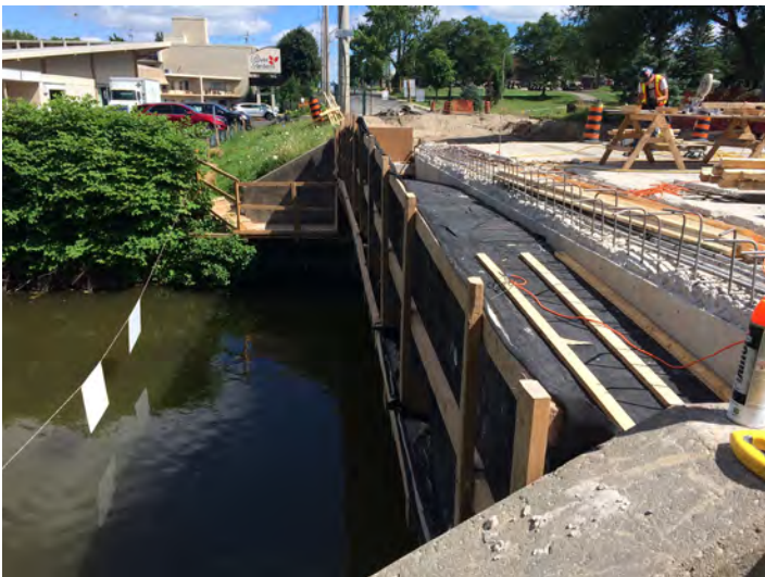
Proper sediment and erosion control measures are in place for this municipal bridge project.
