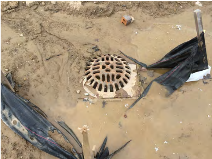
This stormdrain inlet has been overwhelmed with sediment from a construction site.
