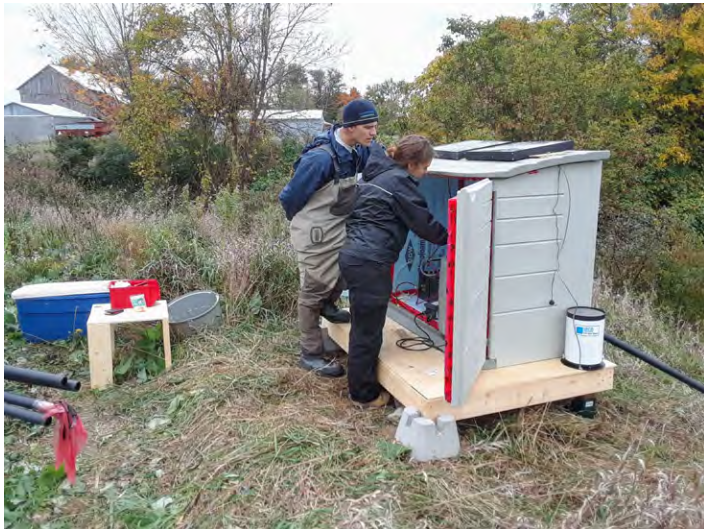
UTRCA staff set up a new water quality monitoring station
