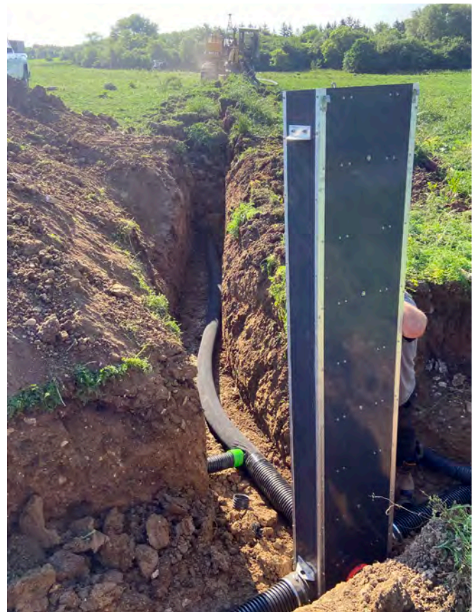
An Agri Drain Inline Water Level Control Structure is installed along this field tile outlet to intercept runoff and direct it into the tile being installed by the drainage plow in the distance.
