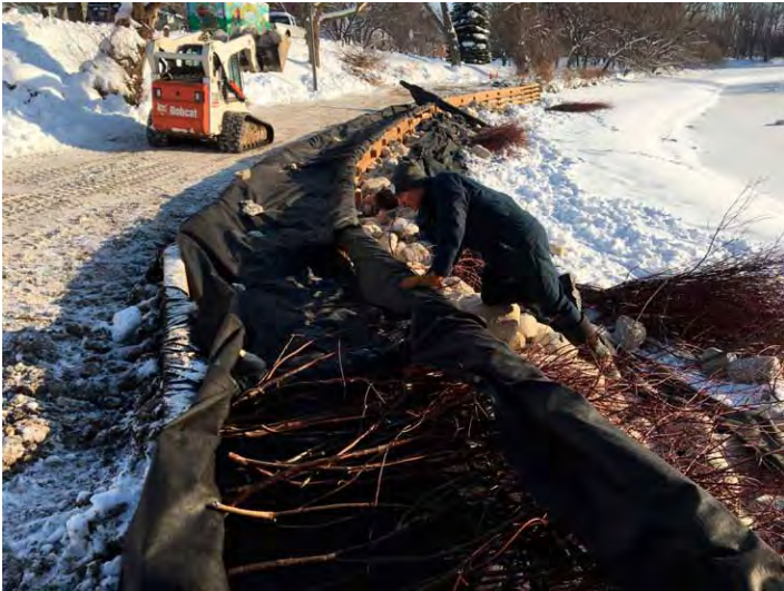
Nearing completion as the filter cloth is placed within the log cribwall.
