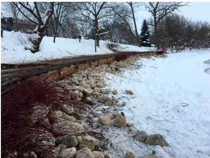
After a bit of final grading, the cribwall is completed and ready for rising water levels and park users.
