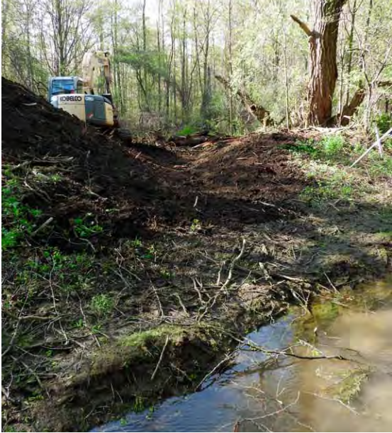
Construction of the trench to reconnect the stream channel to the floodplain.
