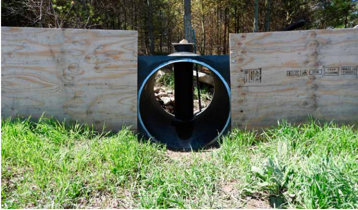
Circular flume for monitoring surface runoff in the Garvey-Glenn Subwatershed
