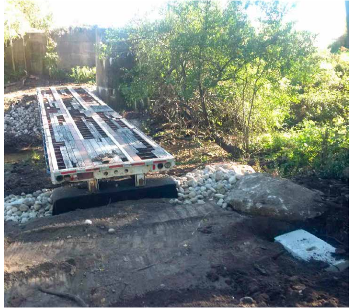
A used truck bed is set in place along the trail. It will be ready for use once the railings, deck boards and lead-up ramps are in place.
