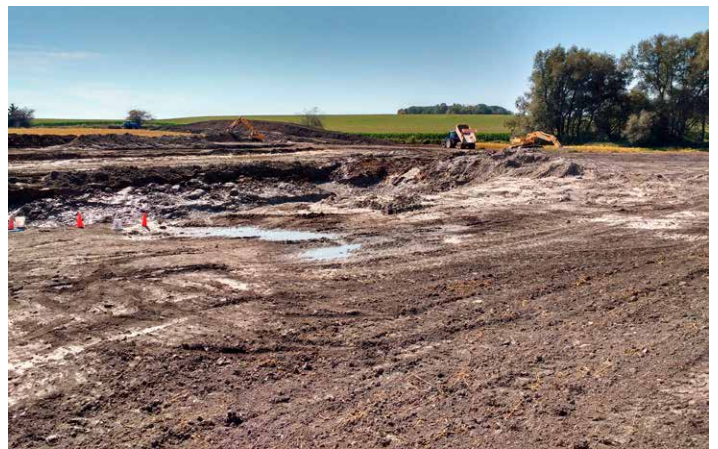
Construction of a 1.5 acre wetland on a retired portion of an agricultural field.
