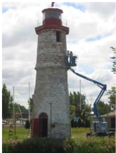
The Thames Lighthouse at Lighthouse Cove on Lake St. Clair received repairs in 2002.
