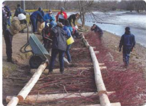
Students and UTRCA staff work on a bioengineering structure in Stratford to protect the bank from erosion.
