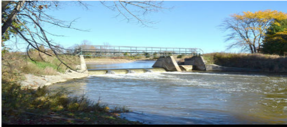
The Lockerby Dam, located in rural Arran Elderslie, between Paisley and Chesley.
