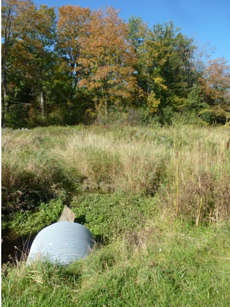
Photo 15. Road culvert on the Neil Drain upstream of Road 163A. A marsh/meadow habitat has established close to the water, with woodland farther back.
