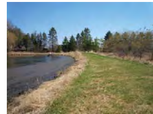
Low earth fill embankment, a grassed, emergency spillway is located at the east end of the embankment. This spillway has a clear width of about 4.0 m and the inlet invert is 0.6 m below the crest of the dam.
