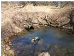
A 762 mm diameter (inner) concrete pipe conveys flow from the pond to a pool at the creek outlet.
