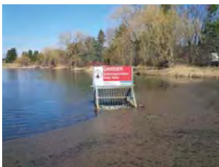
The outlet of the dam includes a concrete bottom draw inlet structure covered with grated trashrack.
