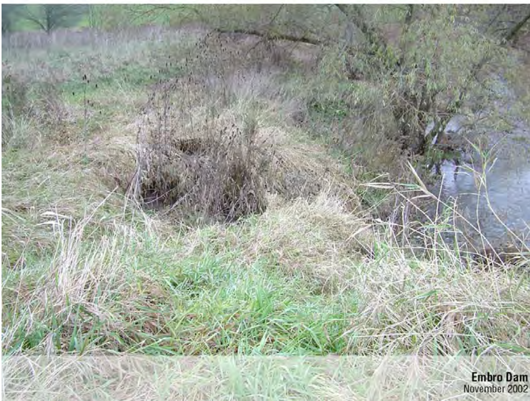
Photo 10 – Eroded Area at Downstream Toe, Left Bank
