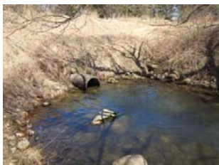
A 762 mm diameter (inner) concrete pipe conveys flow from the pond to a pool at the creek outlet.
