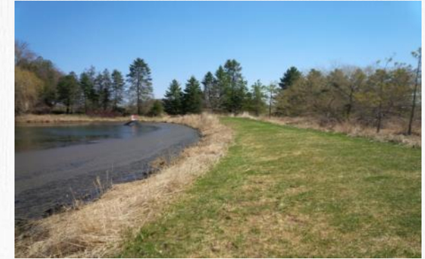
Low earth fill embankment, a grassed, emergency spillway is located at the east end of the embankment. This spillway has a clear width of about 4.0 m and the inlet invert is 0.6 m below the crest of the dam.
