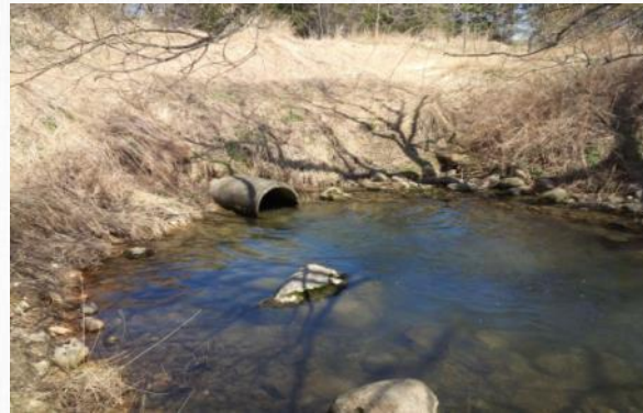
A 762 mm diameter (inner) concrete pipe conveys flow from the pond to a pool at the creek outlet.
