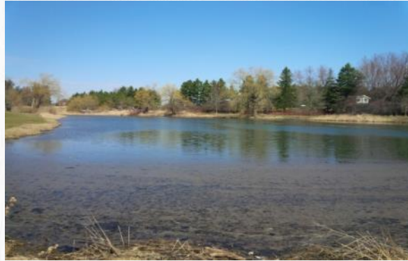
The dam contains water year round and includes approximately 3.4 m of head acting across the dam.
