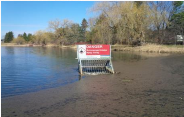
The outlet of the dam includes a concrete bottom draw inlet structure covered with grated trashrack.
