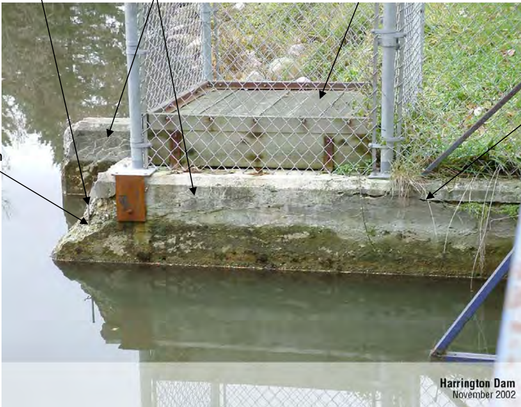
Photo 16 – Concrete Deterioration, Left Abutment
