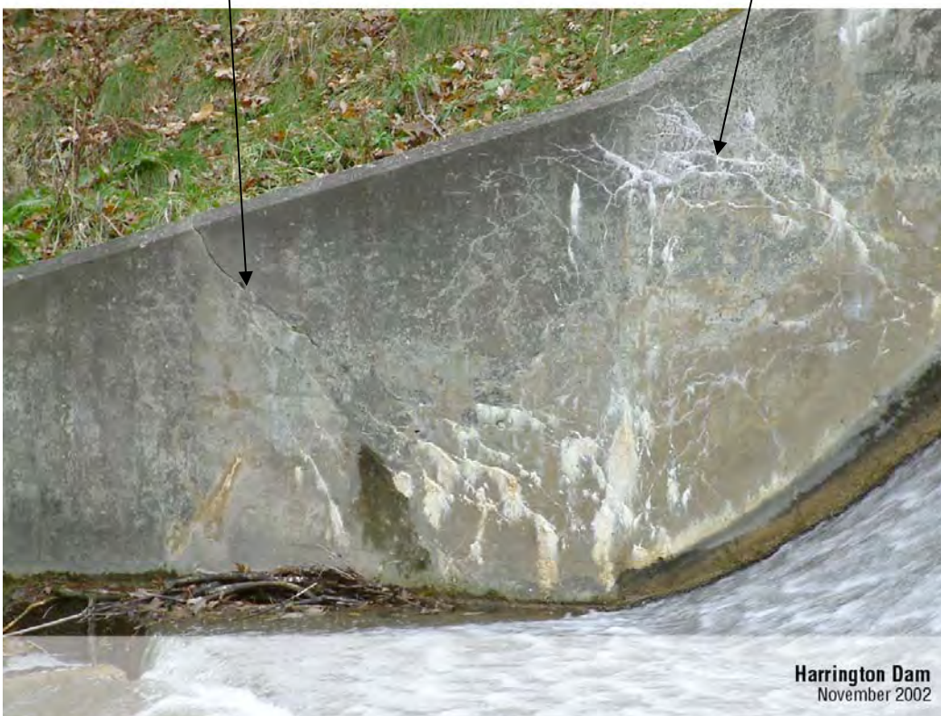
Photo 15 – Close-up of Cracking in Right Downstream Wingwall
