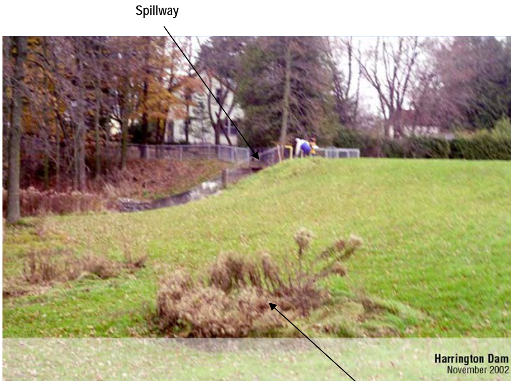
Photo 12 – Leakage Area, Left Downstream Slope
