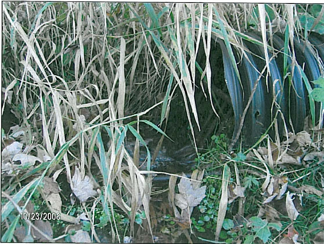
Photo 18: Artesian well outlet pipe located near twin box culvert.
