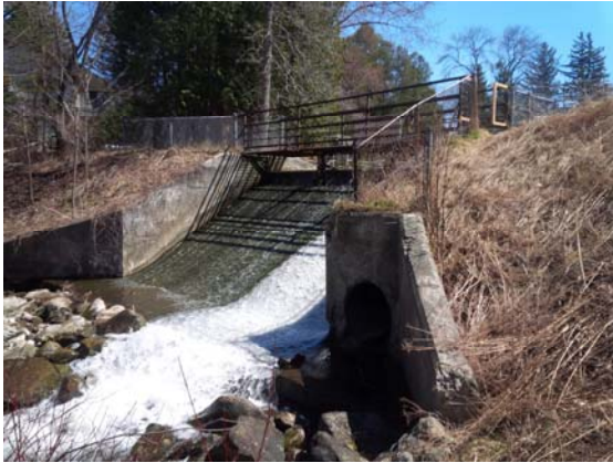
The Harrington Dam is approximately 90m to 95m long, with two earthen embankments flanking a concrete spillway.
