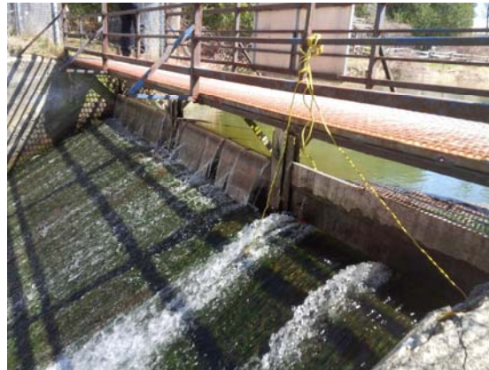
The dam spillway is considered to have an inadequate capacity for safety and stability purposes; the water level in the reservoir can be adjusted by adding stop logs to the spillway.
