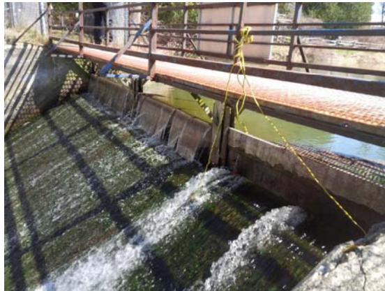
The dam spillway is considered to have an inadequate capacity for safety and stability purposes; the water level in the reservoir can be adjusted by adding stop logs to the spillway.
