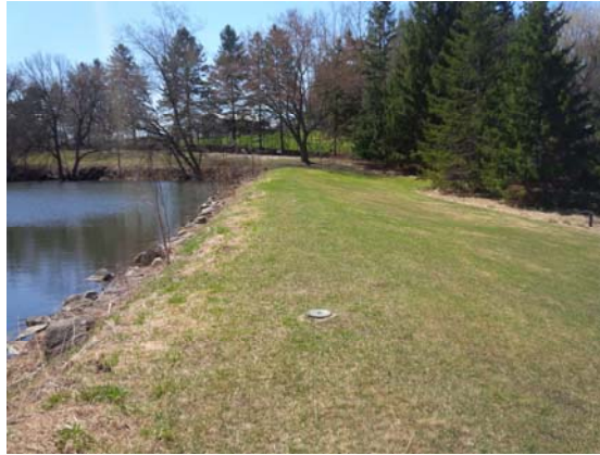
The earthen embankments of the dam are founded on soil overburden, rather than bedrock or engineered soil.
