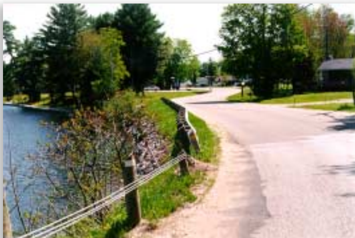
Figure 81 - Bent Guardrail Due to Failure Below Water Line
