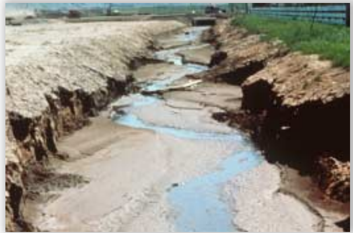
Figure 99 - Example of 'Active' Bank Erosion
