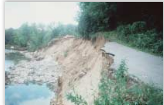
Figure 31 - Manmade Hazard Damages
