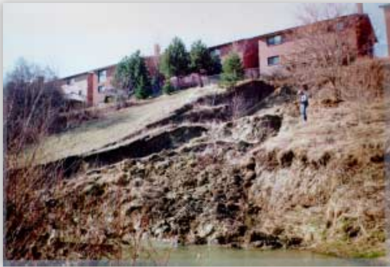
Figure 1 - Slope Slide Caused By River Erosion
