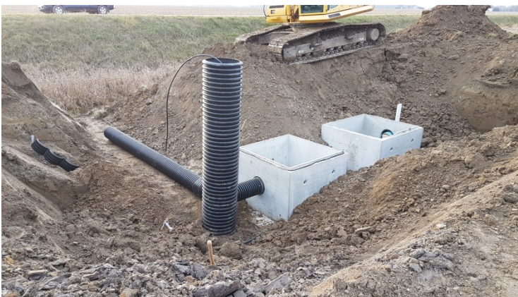
Installation of the Phosphorus Treatment Tank in November of 2017 photo credit: LTVCA)
