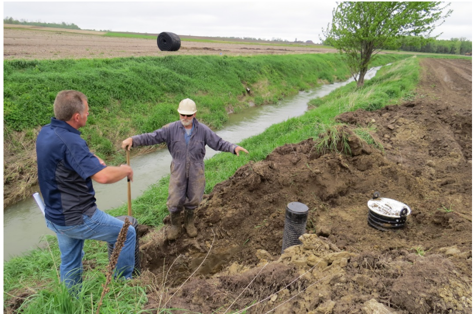
UTRCA's Brad Glasman (Manager of Conservation Services) installing a controlled drain with a landowner (photo credit: UTRCA)
