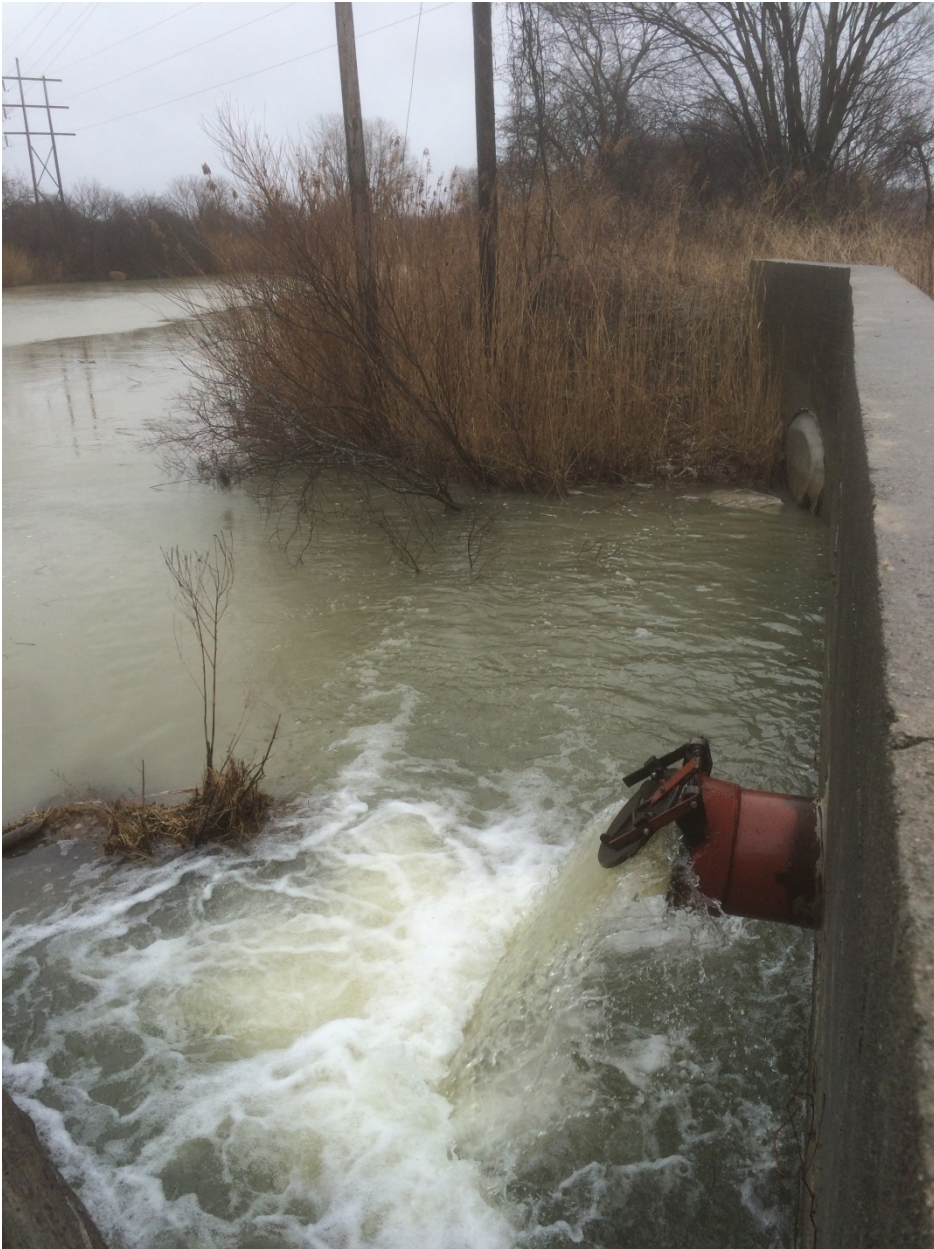
Jeannettes Creek Boudreau Pump Station operating during a melt event in March of 2016 (photo credit: LTVCA)
