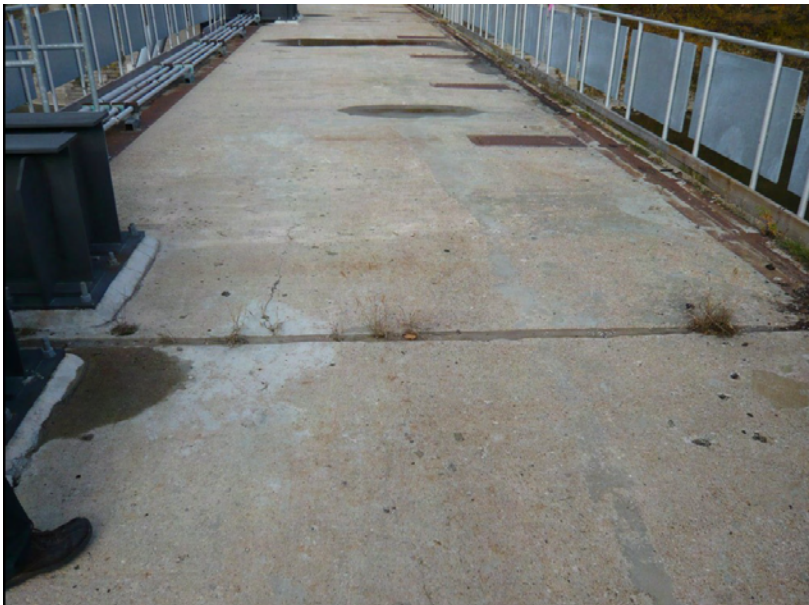
Photo 16: Springbank Dam bridge deck, looking north. Note the holes in the concrete for the old gate guides (welded shut by thin plates).
