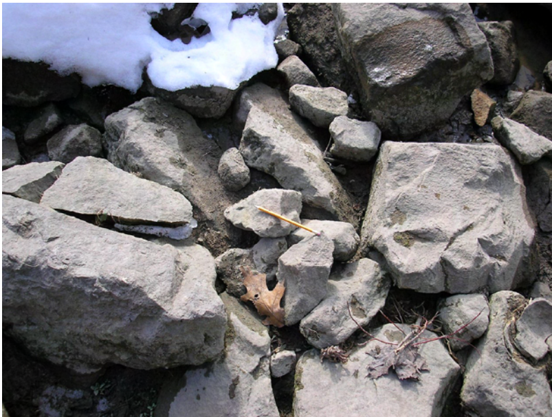
Photo 14: Riprap protection at the upstream side of the crib (stone diameter varies from 0.1 to 1.0 m). Some cracking in the stones is evident, but the riprap is in generally good condition
