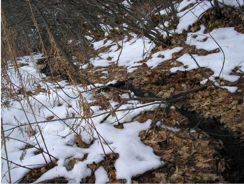
Photo 11: Toe of slope downstream of the dam, standing on top of crib. Seepage from the slope is seen to drain in a small channel that eventually empties at the downstream side of the crib
