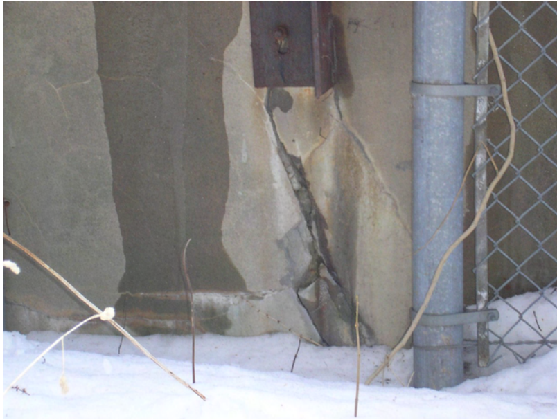
Photo 19: Vertical crack adjacent to the fence post on the north end of the deck.
