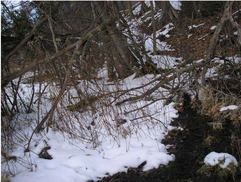
Photo 12: Toe of slope upstream of the dam, standing on top of crib. Again seepage from the slope drains in a less defined channel (due to trees) and eventually empties at the upstream side of the crib
