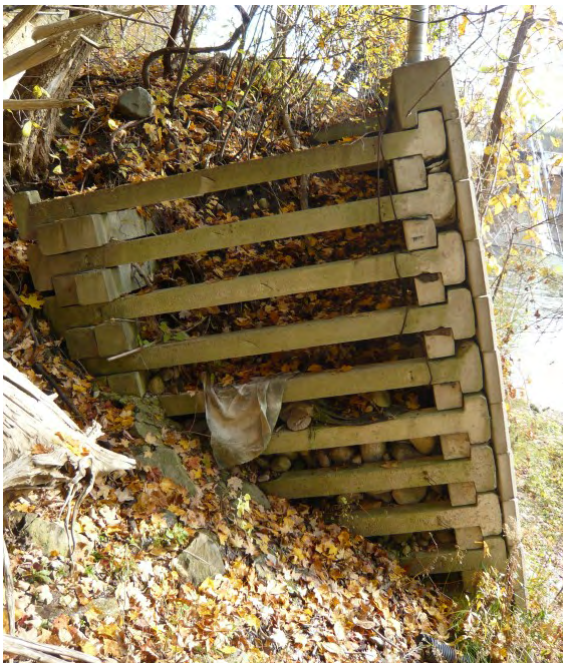
Photo 4: Downstream end, material lost due to surface runoff and erosion.
