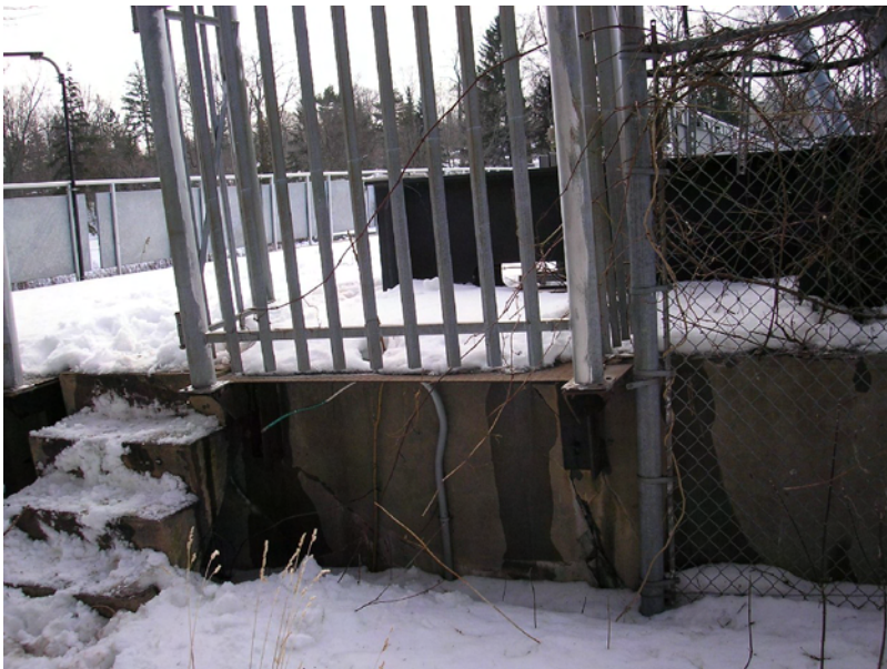
Photo 18: North end of the deck, vertical cracks are observed adjacent to the stairs and adjacent to the fence post.
