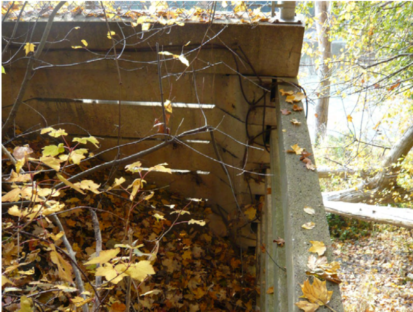
Photo 3: Downstream end of the crib. Note the material lost.
