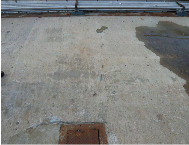
Photo 17: Typical view of the deck slab at the old gate guides (looking downstream). Note the crack running along the length of the slab from the pipes to the old gate guides (see pen for scale).
