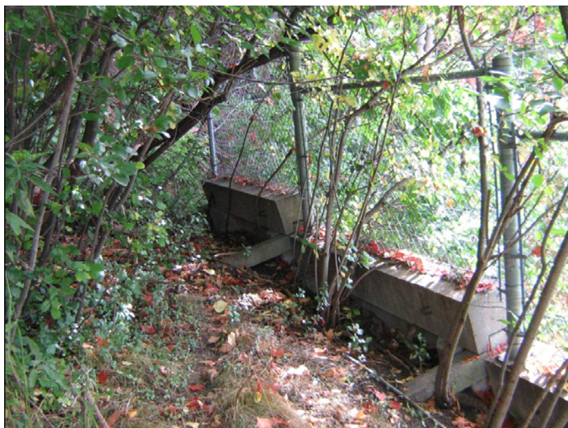
Photo 10: Top of crib on the upstream side of the crib, looking upstream. Shown in the figure is material eroded from top of the crib.
