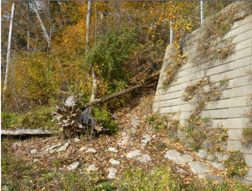
Photo 1: North embankment crib, downstream portion (standing on bottom and looking downstream). Most of the surface runoff flows bypasses the crib.
