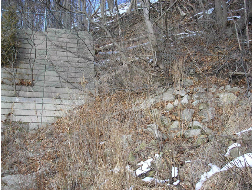
Photo 5: Upstream return portion of the crib, showing the upstream extent of riprap.
