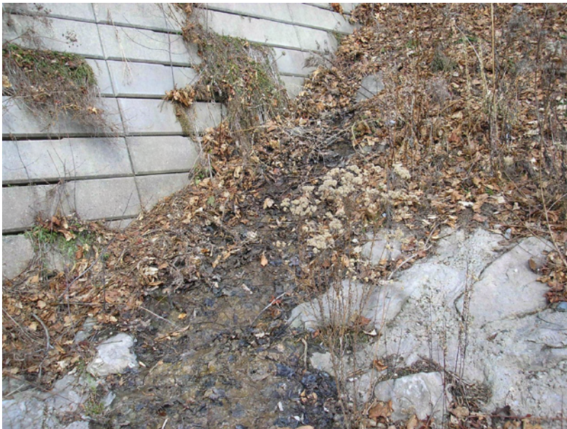
Photo 6: Slope at the upstream end of the crib, showing runoff from the top of the crib
