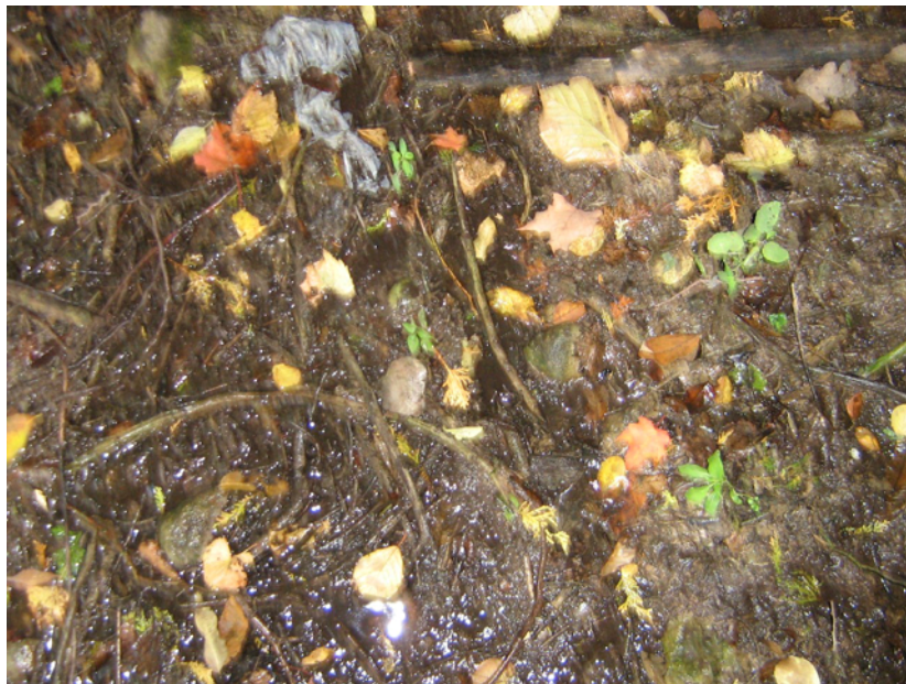
Photo 9: Puddles and pools on the fill material on top of the crib
