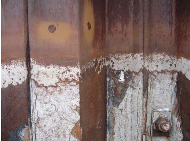
Photo #7 – Prepared surface for steel sheet pile thickness measurement at location T1 above high water mark.
