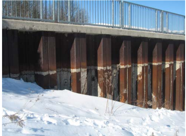
Photo #2 –Front Elevation, east end of wall at embankment. High water mark visible.
