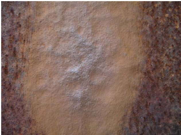
Photo #9 – Prepared surface for thickness measurement at location on T4 & T5 steel sheet pile web.
