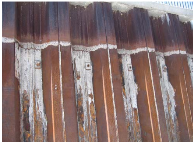
Photo #6 – Tie rod shown every third inpan. Heavy corrosion below high water mark.
