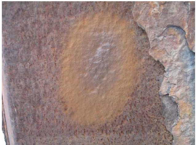
Photo #10 – Prepared surface for thickness measurement at location on T8 on web with rust scale to the right.
