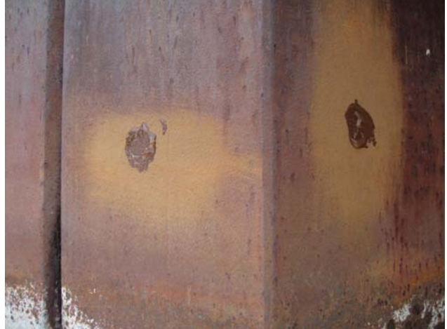
Photo #8 – Close up of prepared surface for thickness measurement at location T1 & T2.
