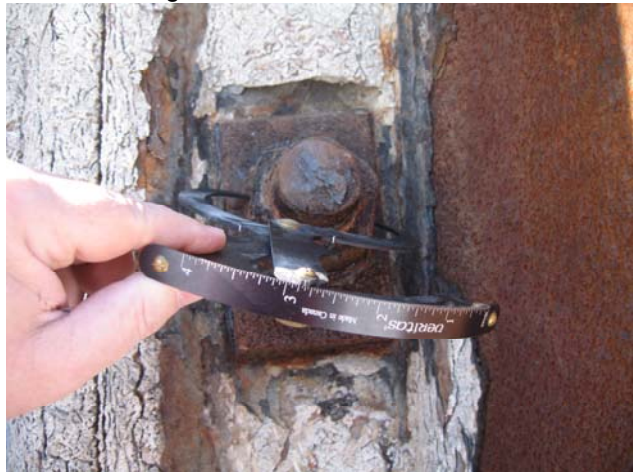
Photo #12 – Measurement across the flat on tie rod nut #7.
