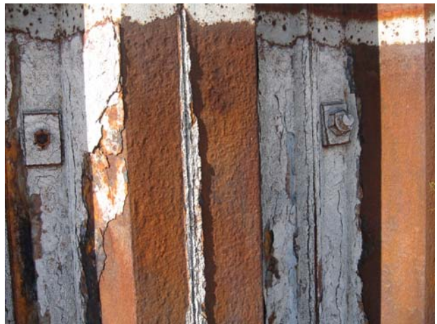
Photo #4 – Evident corrosion and pitting on face of outpans. Rust scale on inpans and partially on webs and interlocks.
