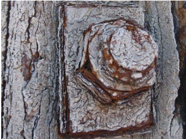
Photo #11 – Typical corroded tie rod, tie rod nut and bevelled washer at tie rod #7.
