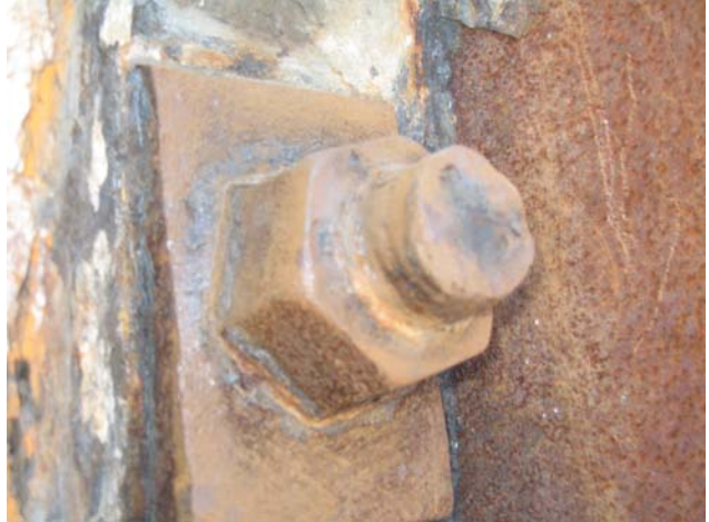
Photo #14 – Tie rod nut and assembly clean of rust scale. Tie rod thread root and crest rounded and barely visible.
