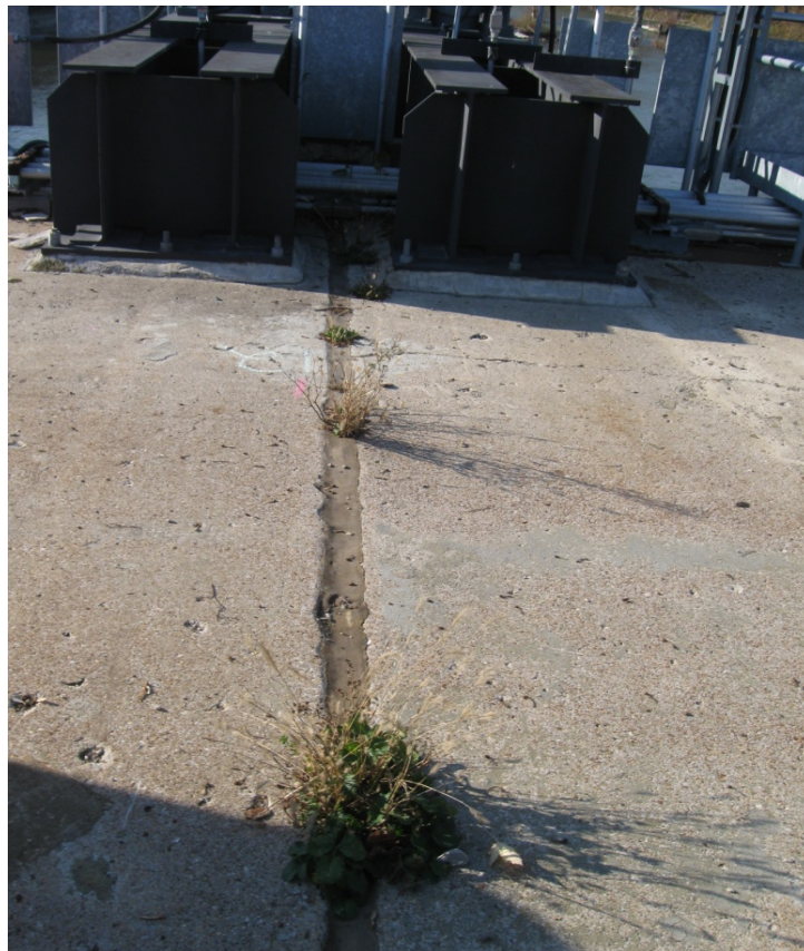
Photo 7 – Vegetation growth in the expansion joint sealant
