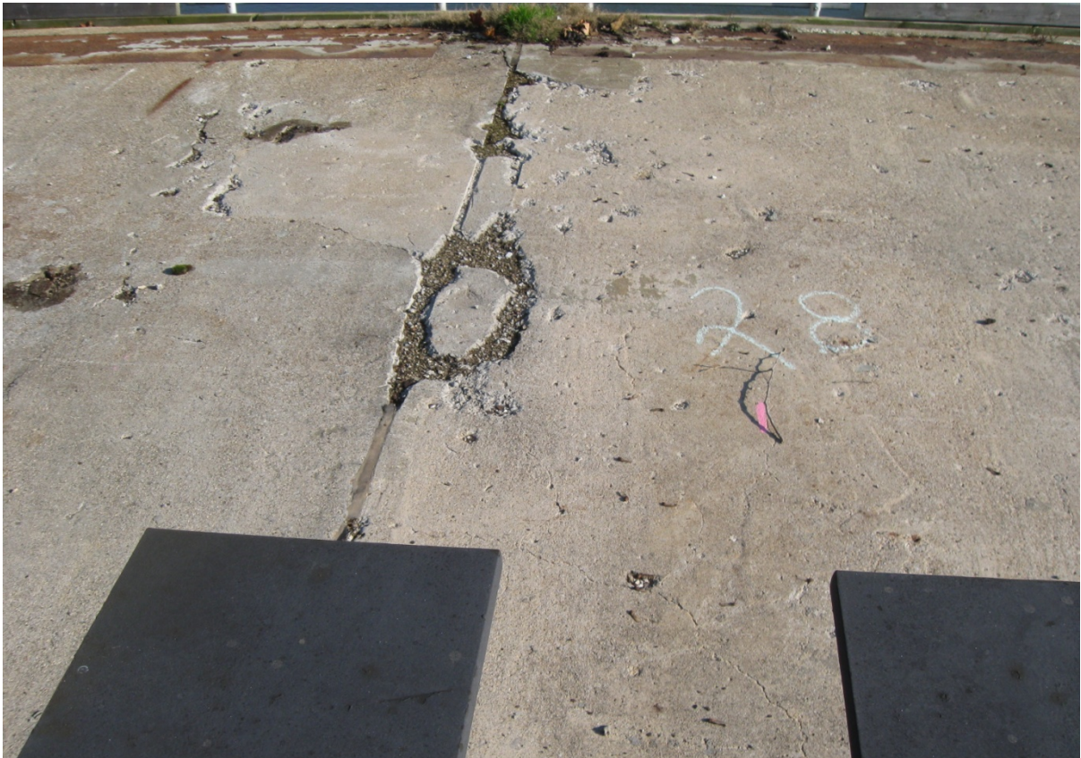
Photo 6 – Spalling at deck joints
