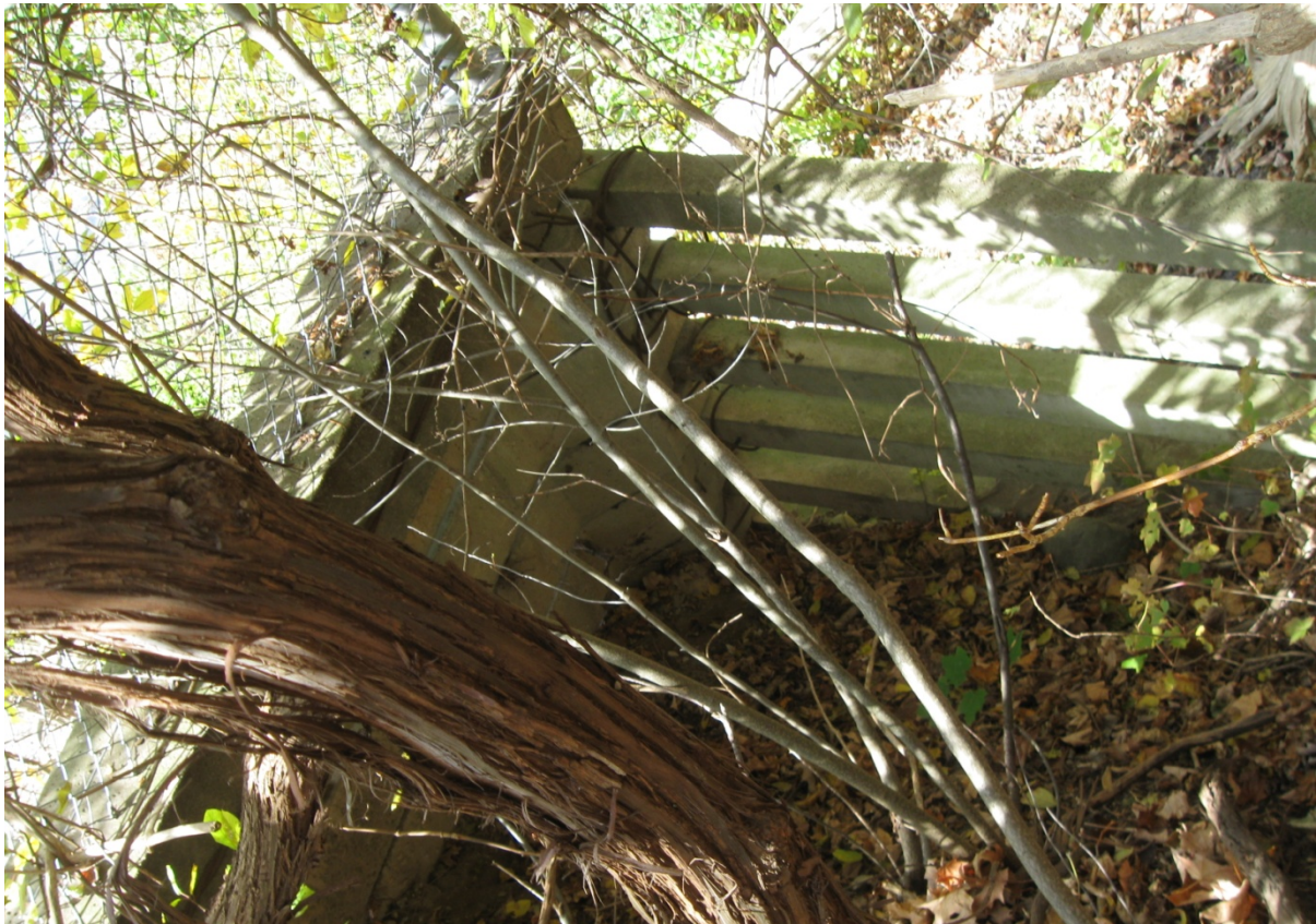
Photo 26 – Erosion behind northwest retaining wall
