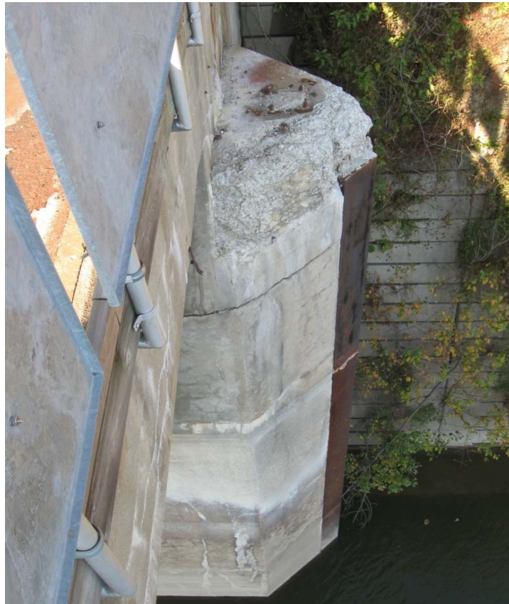
Photo 22 – Severe scaling top of north pier, upstream side
