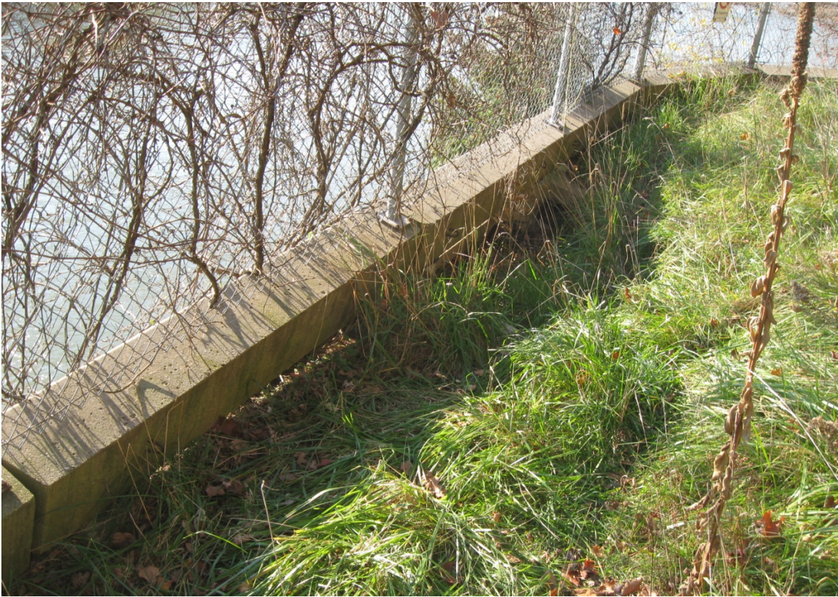
Photo 25 – Erosion behind northwest retaining wall
