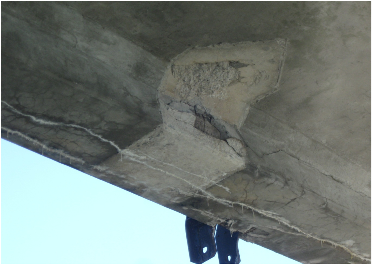
Photo 9 – Close-up of spalling at south span
