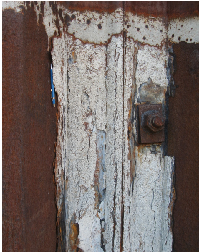
Photo 29 – Severe flaking of southeast retaining wall
