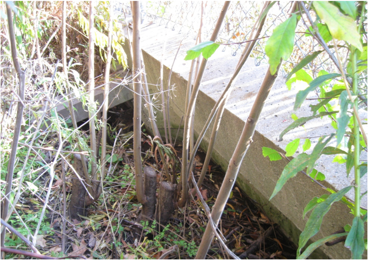
Photo 27 – Erosion behind northeast retaining wall
