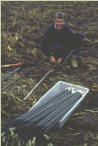
Installing peizometers to test nitrate movement on an Embro area farm, UTRCA
