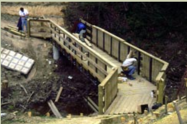
Conservation Authority staff work on a new bridge for the Thames Valley Trail in Fanshawe CAM
