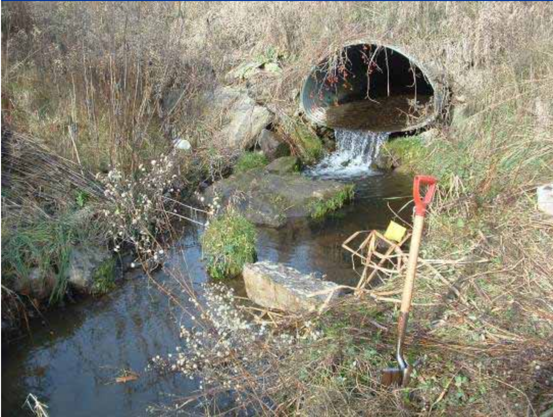
1. Perched culvert barrier
