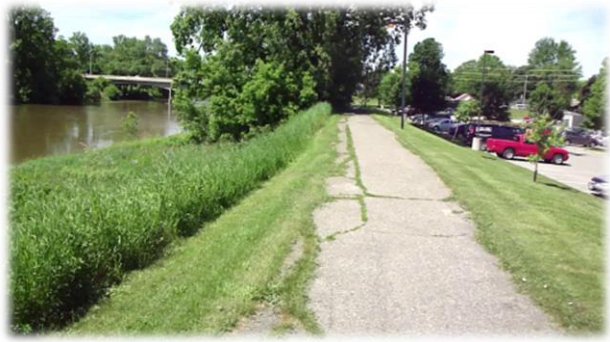
Figure 4.17: Wharncliffe Berm (Near Kiwanis Seniors' Community Centre, Facing West)
