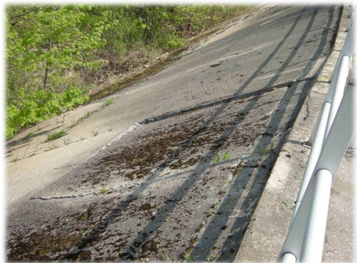
Figure 10.2: Panel Deficiency Noted During Inspection
