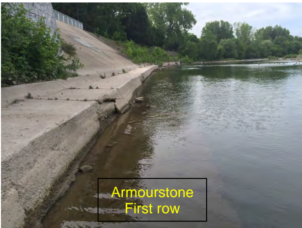
Photo 2-5 – Leslie Street Site looking upstream at right bank and deepest area of scour pool. The first row of armourstone (submerged) is in good condition. Some of the blocks from the second row (at right, not visible) have fallen into the pool. View upstream.
