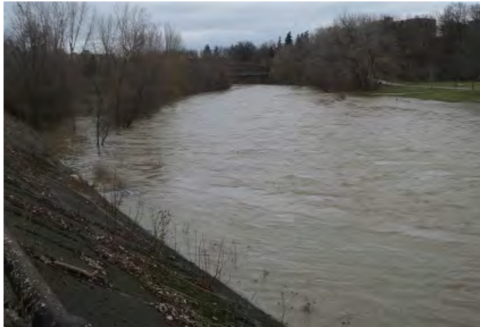
Photo 2-3 – Leslie Street Site (Vantage 1), April 10, 2015. River discharge 157.7 m 3 /s. Flows near to toe of the dyke are relatively calm, with no indication of excessive turbulence or scour.
