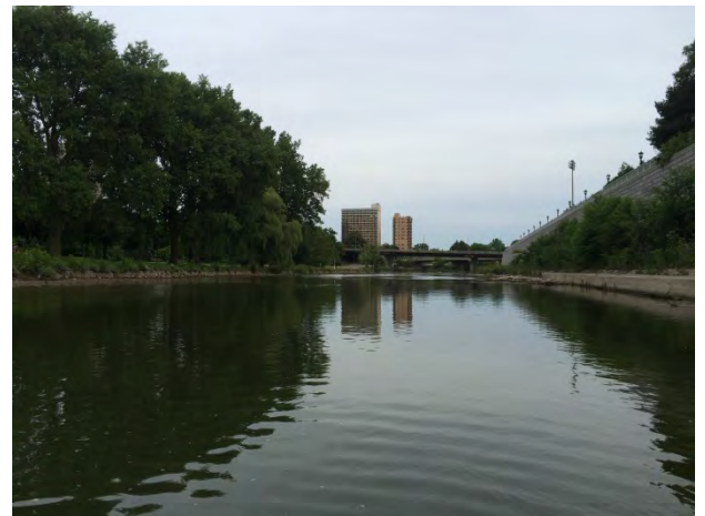
Photo 2-6 – Leslie Street Site looking at downstream riffle. Gabion baskets along left bank were failing.
