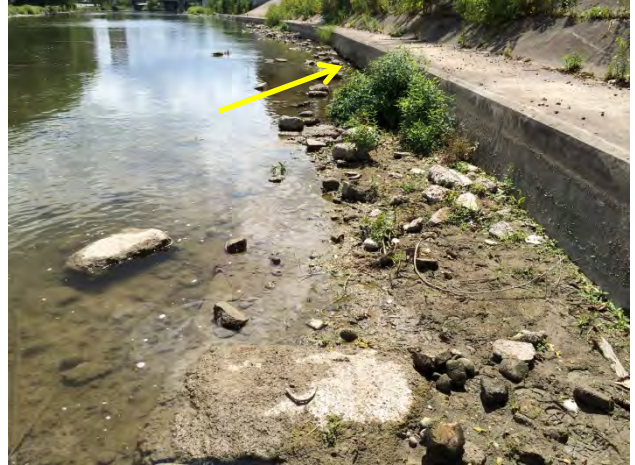
Photo 2-2 – Leslie Street. Base of dyke and armourstone toe along the upstream section of the compound pool. Sections of the concrete toe of the dyke have been undermined (arrow). View downstream.
