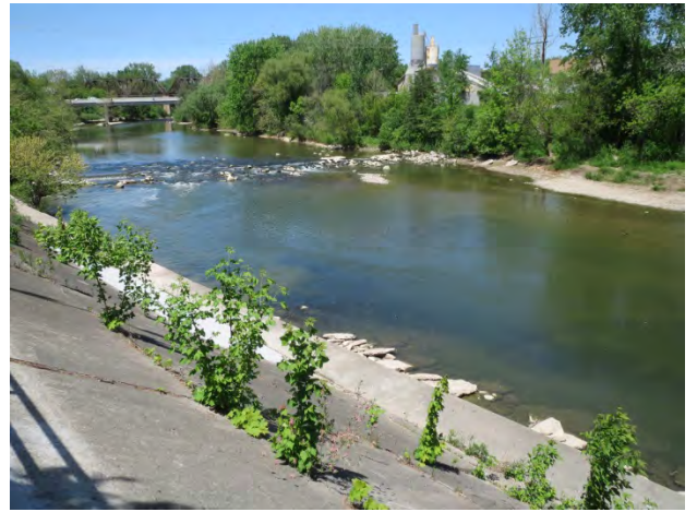
Photo 1-4 – Ann Street Weir, May 20, 2015. River discharge 3.1 m 3 /s. Turbulence evident along dyke toe despite low flows.
