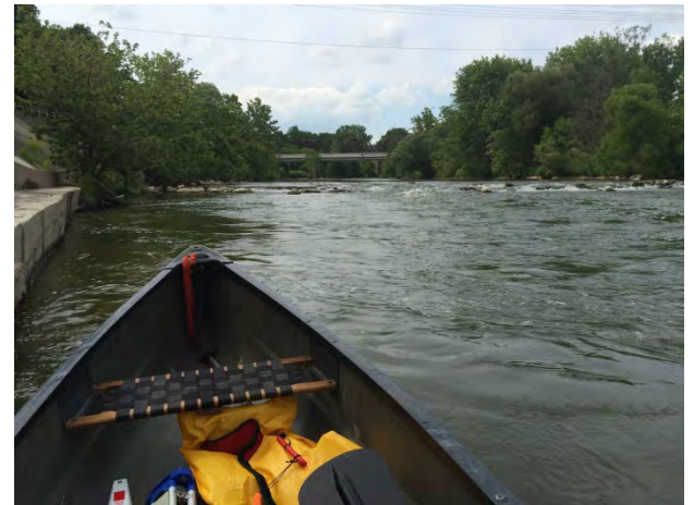
Photo 1-6 – Downstream of Ann Street Weir looking upstream at right bank scour pool. Note eddying effect at location of scour pool.
