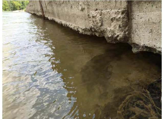
Photo 1-2 – Ann Street Site. Dyke toe 25 m downstream of weir showing 0.4 m undercut. The substrate (submerged) is silt till. View downstream.
