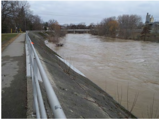
Photo 1-3 – Ann Street Weir, April 10, 2015. River Discharge 157.7 m 3 /s. Frequent boils visible on the water surface at the toe of the dyke indicate turbulence (kolks) and high shear.
