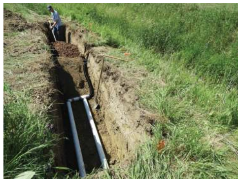
Step 2: Underdrains installed at the bottom of trench to drain the biofilter
